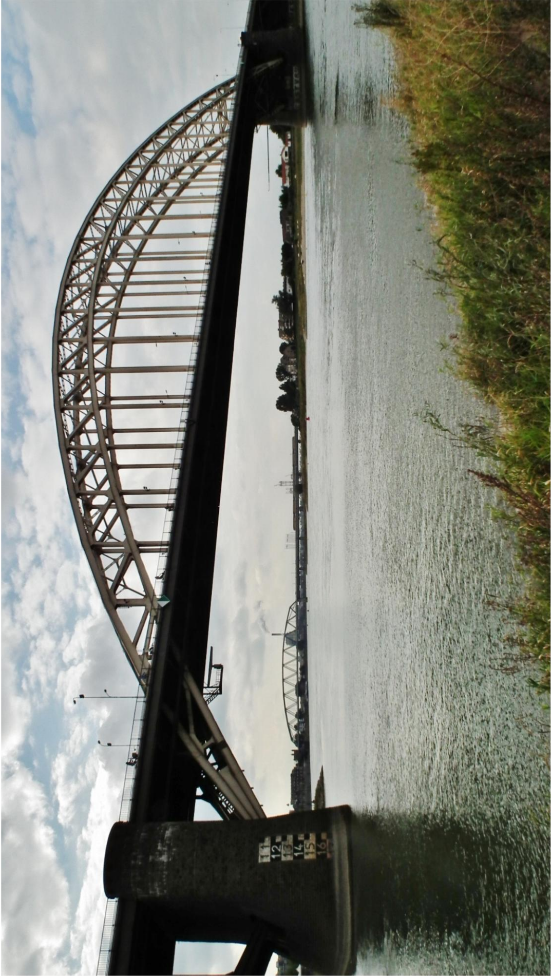
This current view of the two bridges, taken from the eastern side of the original road bridge, shows the repaired rail bridge. The damaged central span and northern arch have been replaced with a single level concrete section.
